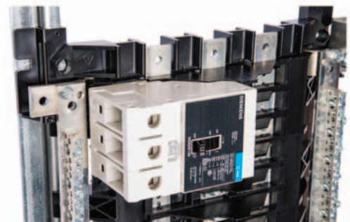
Example of Back-fed xGB Main breaker installed
