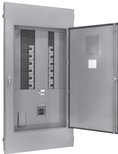
Access to Circuit Breaker Handles
