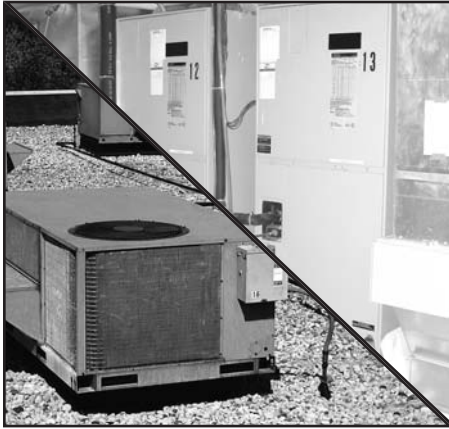
HVAC Equipment Split System
